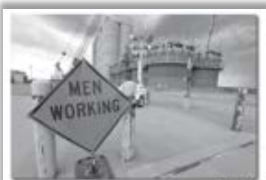
An 811 utility operator at the New Century job site. The sign is a warning to anyone who might be digging in the area.
